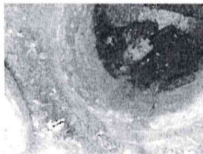
Manhole Defect Photos:
