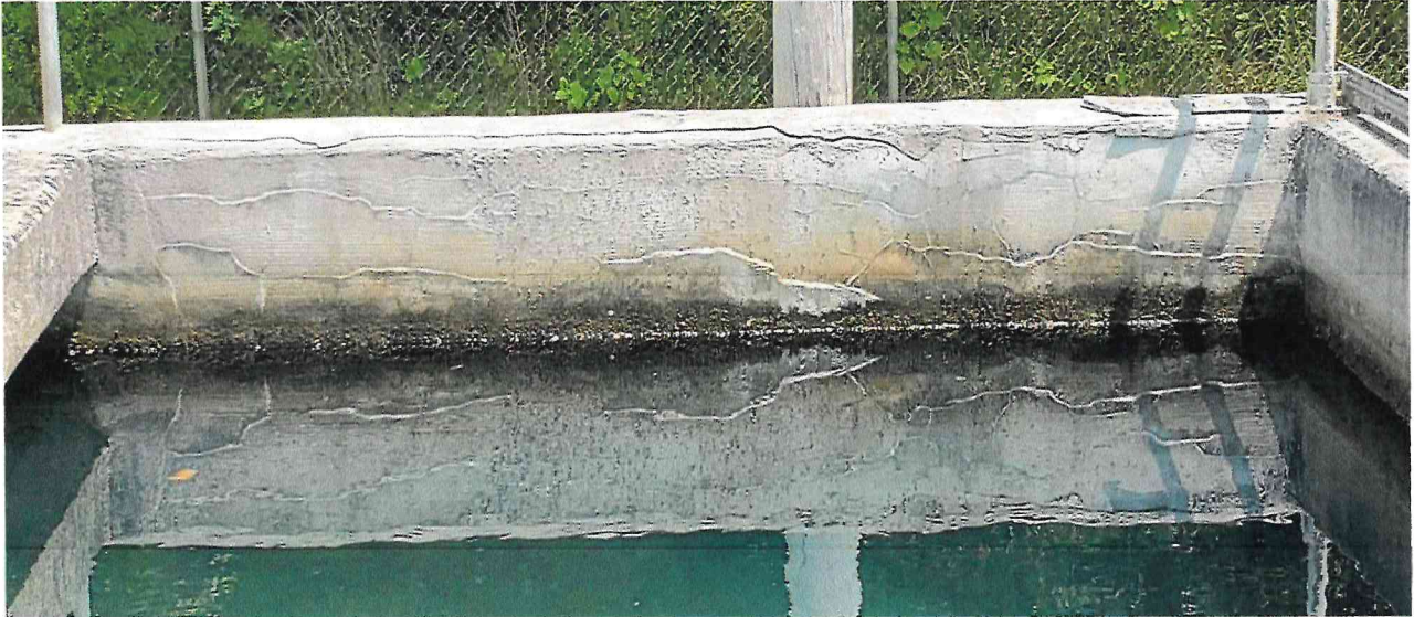
Figure – 2 Monteagle Water Plan – Headworks Wall – Damage/Deterioration
