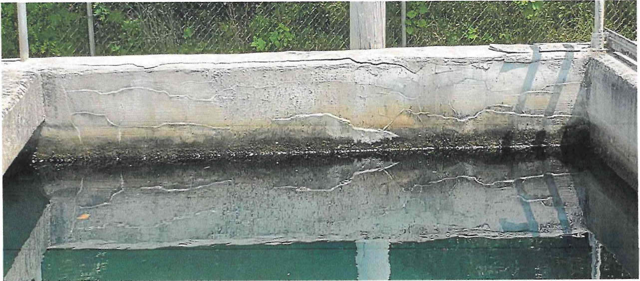
Figure – 2 Monteagle Water Plan – Headworks Wall – Damage/Deterioration
