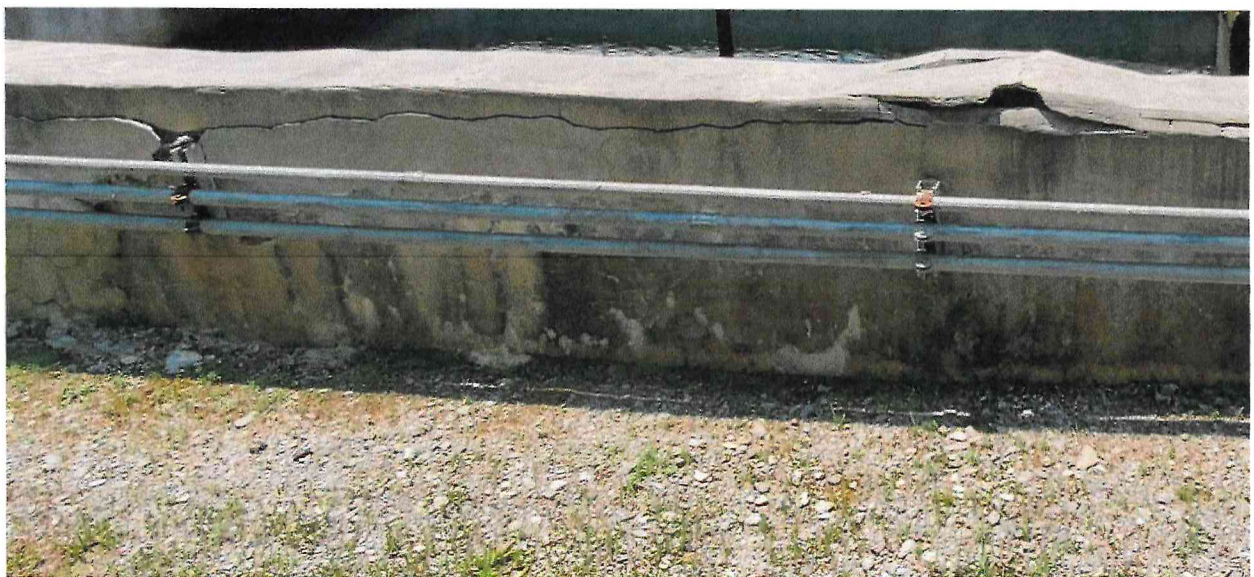
Figure – 1 Monteagle Water Plan – Headworks Wall – Damage/Deterioration
