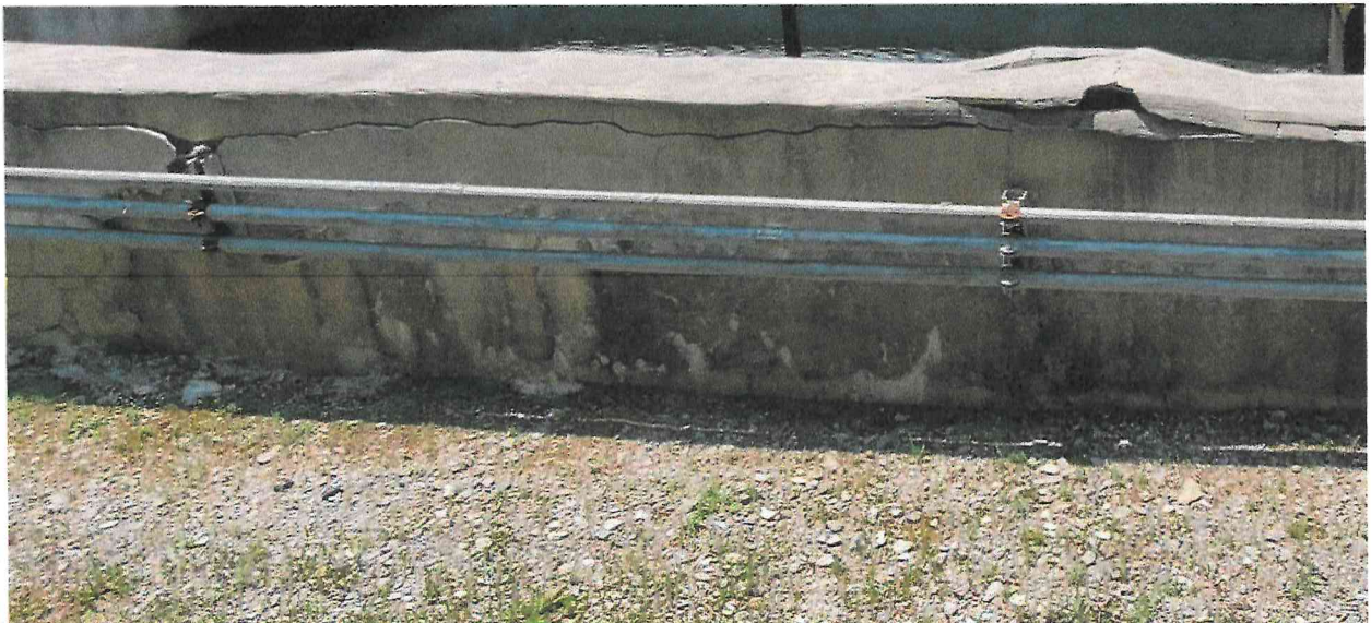
Figure – 1 Monteagle Water Plan – Headworks Wall – Damage/Deterioration
