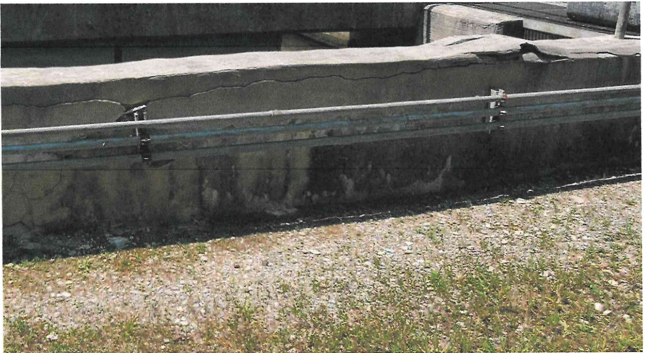
Figure – 3 Monteagle Water Plan – Headworks Wall – Damage/Deterioration
