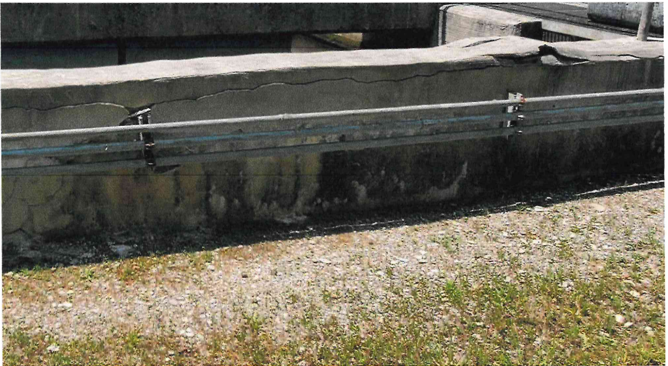
Figure – 3 Monteagle Water Plan – Headworks Wall – Damage/Deterioration
